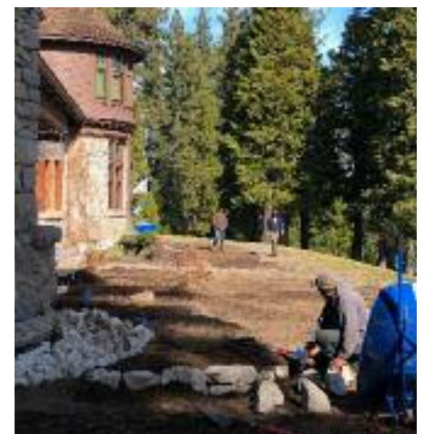
Landscape Restoration work at Pine Lodge. SSPF is restoring the garden to its 1964 appearance and installing a barrier to protect the structure and reduce run-off into Lake Tahoe.
